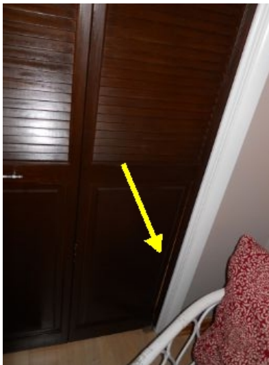
Closet door is broken
