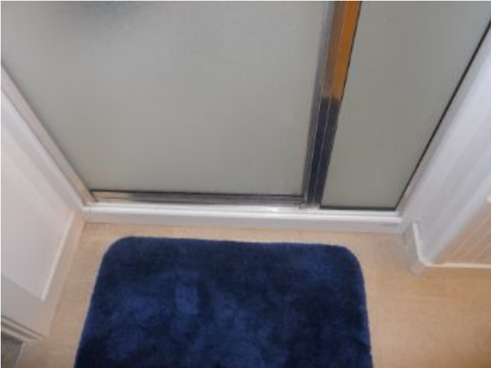
Some water stains noted
