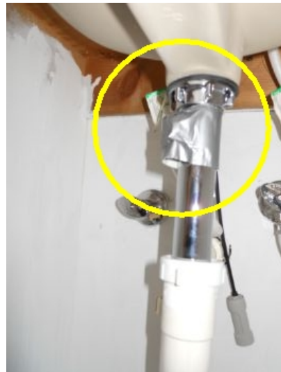
Sink drain has been patched with Duct Tape
