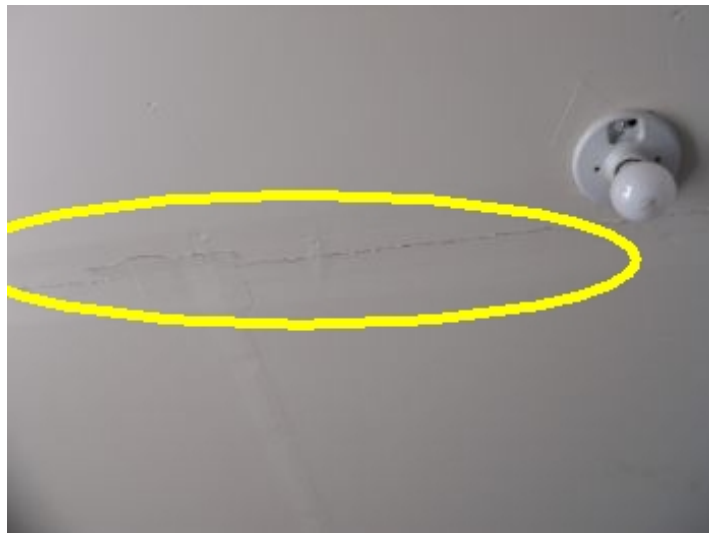
Fire Taping needs to be repaired
