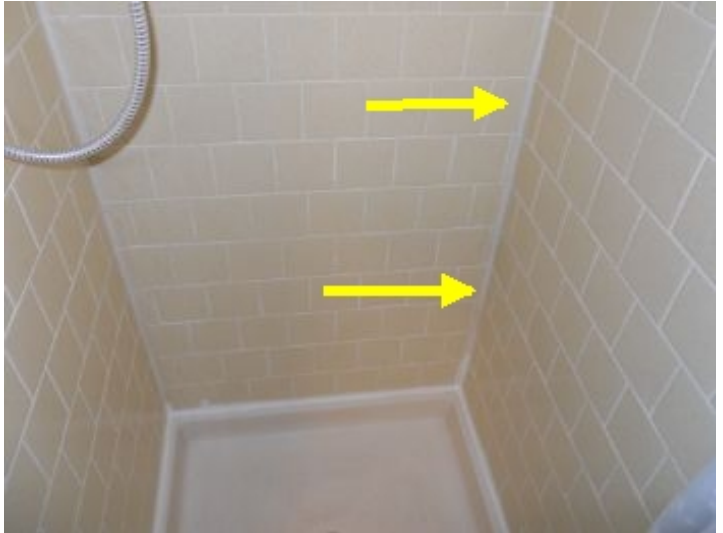
excessive caulk used to seal shower
