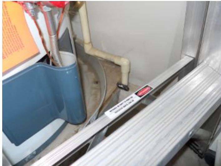
bracket needs to be re-attached
