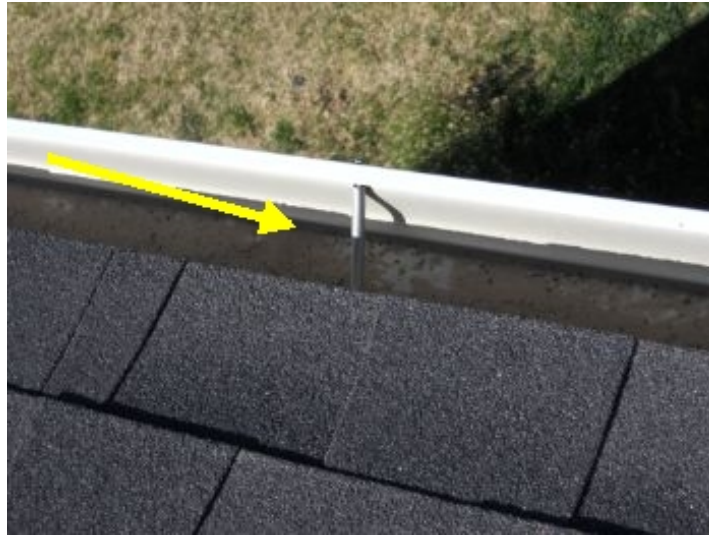
Few Nails need re-attached
