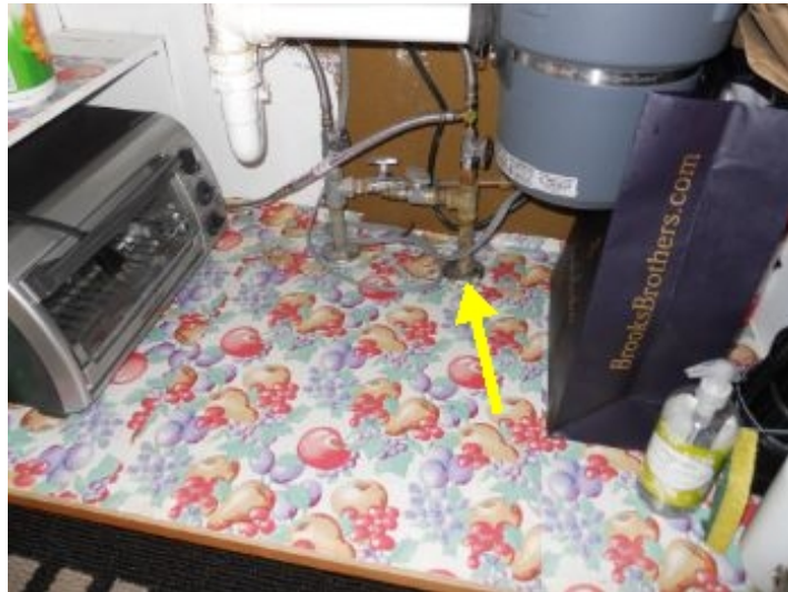
Evidence of past leaks
