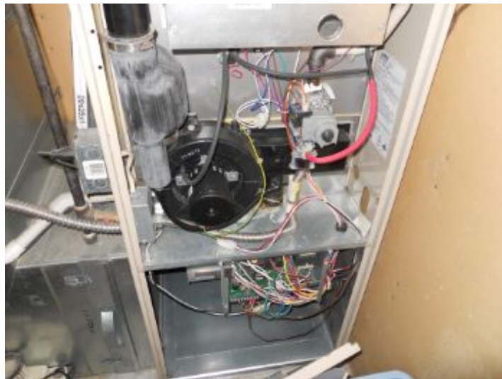
Furnace operates and looks in good condition
